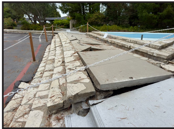
Concrete and stone stairs buckling due to the increasing speed of the Portuguese Bend landslide.
