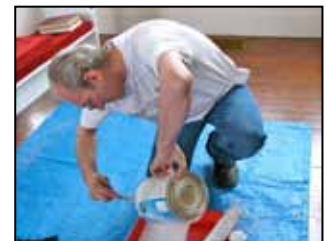
Rick Cruz spearheaded installing the new sanctuary carpet and painting the pews.
